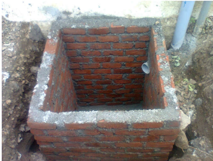
Underground Collection Tank for collecting Rain Water
