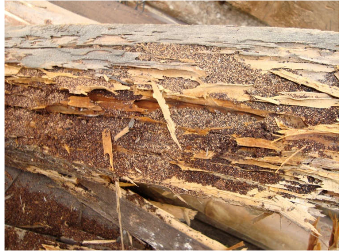
Figure 4. Damage caused by the action of termites of the species Cryptotermes brevis on the wooden roof rafters in the Raft Room at the National Museum of the Sea, São Francisco do Sul, SC. Ceiling lying on the floor
