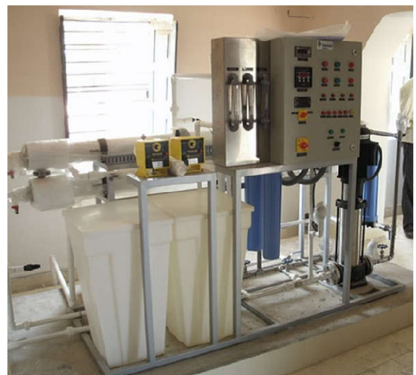
Figure 6. Reverse Osmosis Plant
