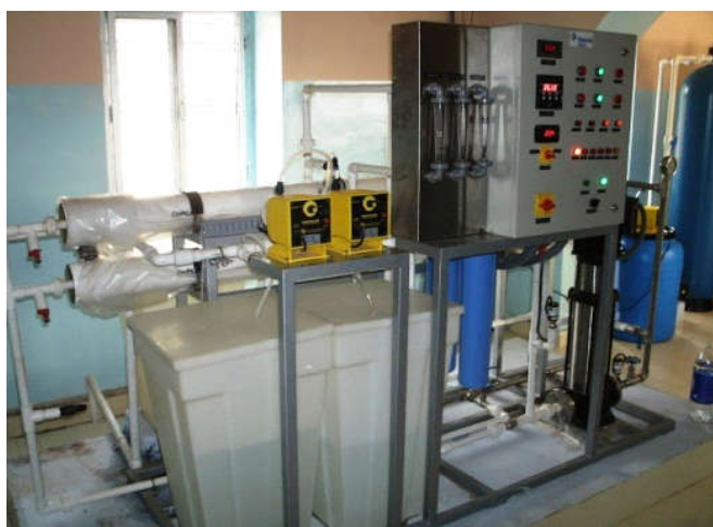
Figure 16. RO Water Treatment Plant installed by Safe Water Network
