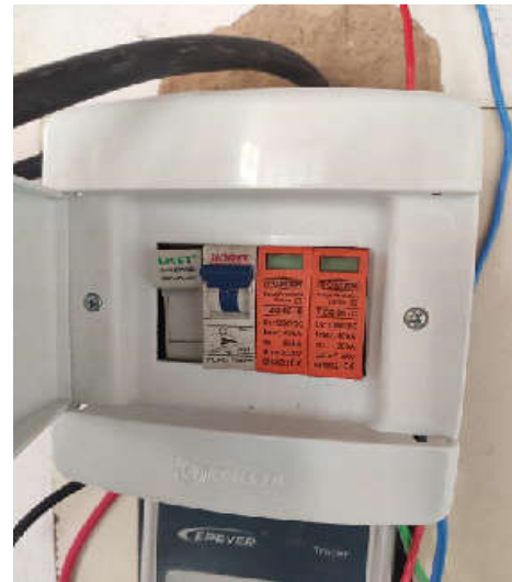
Fig. 7. Electrical protective box
