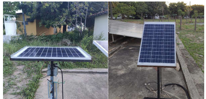
Fig. 3. Two photovoltaic modules installed
