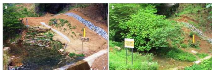
Figure 6. Evolution of soil bioengineering work. a Work immediately after execution in August 2014; b Intervention after 16 months.
