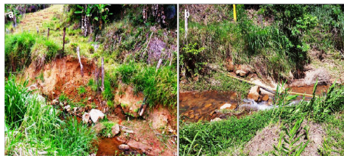
Figure 1. Stream after erosion processes with unstable bed and banks. a Landslide at the left side of the streambank; b Detail of exposed fiber the optical cables
